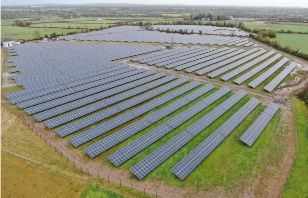
Bullstown Solar Farm Overview
